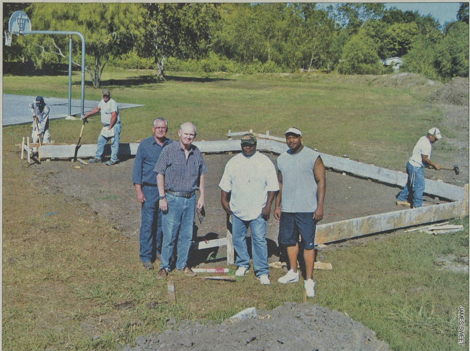
Kevin Earls (second from right) and Jerome McAfee (far right) representing Old Skool, Thurston Webb, Public Works Director, (far left) and City Councilman Mike Cooper (second from left) look on as employees of Class Concrete complete the form for the new rest room facility at the city's E. H. Henry Park. In support of the project, Jimmy and Barbara Class of Class Concrete donated the concrete, labor, and form material.
